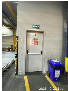
Emergency exit door.JPG
