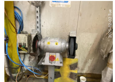
NC-No face guard for grinding machine.JPG
